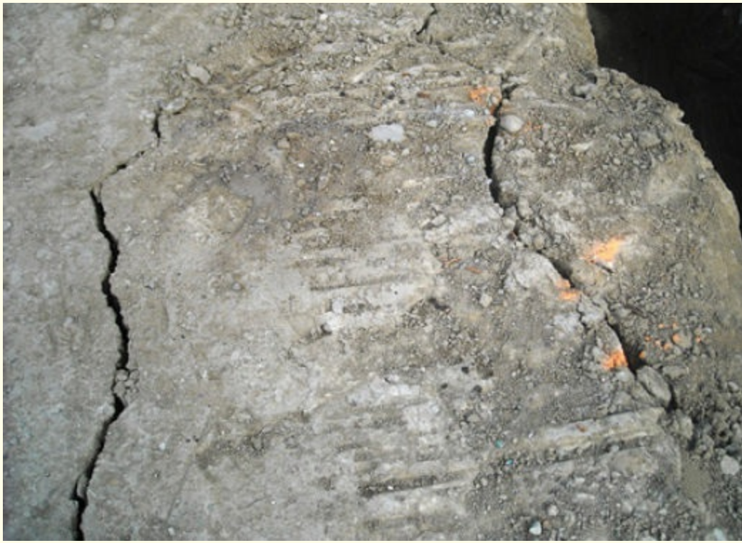
FIGURE 3-9 Cracks in the soil indicate drying and can be the first sign of faults in and around the open trench. Courtesy of Ron Zawlocki
