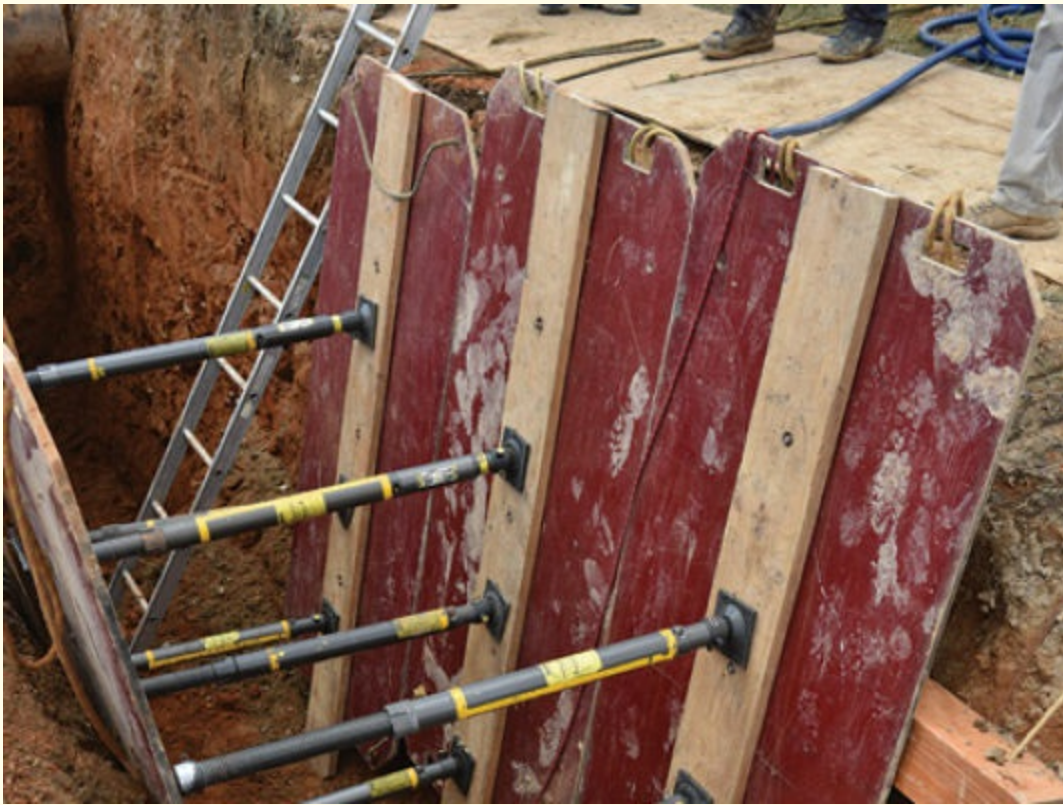
FIGURE 10-13 Outside wales are used to span a slough in the trench wall.
