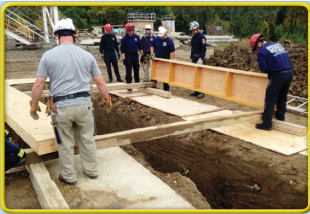
3 Place decking on the girders and slide the decking to the edge of the trench. Courtesy of Ron Zawlocki
