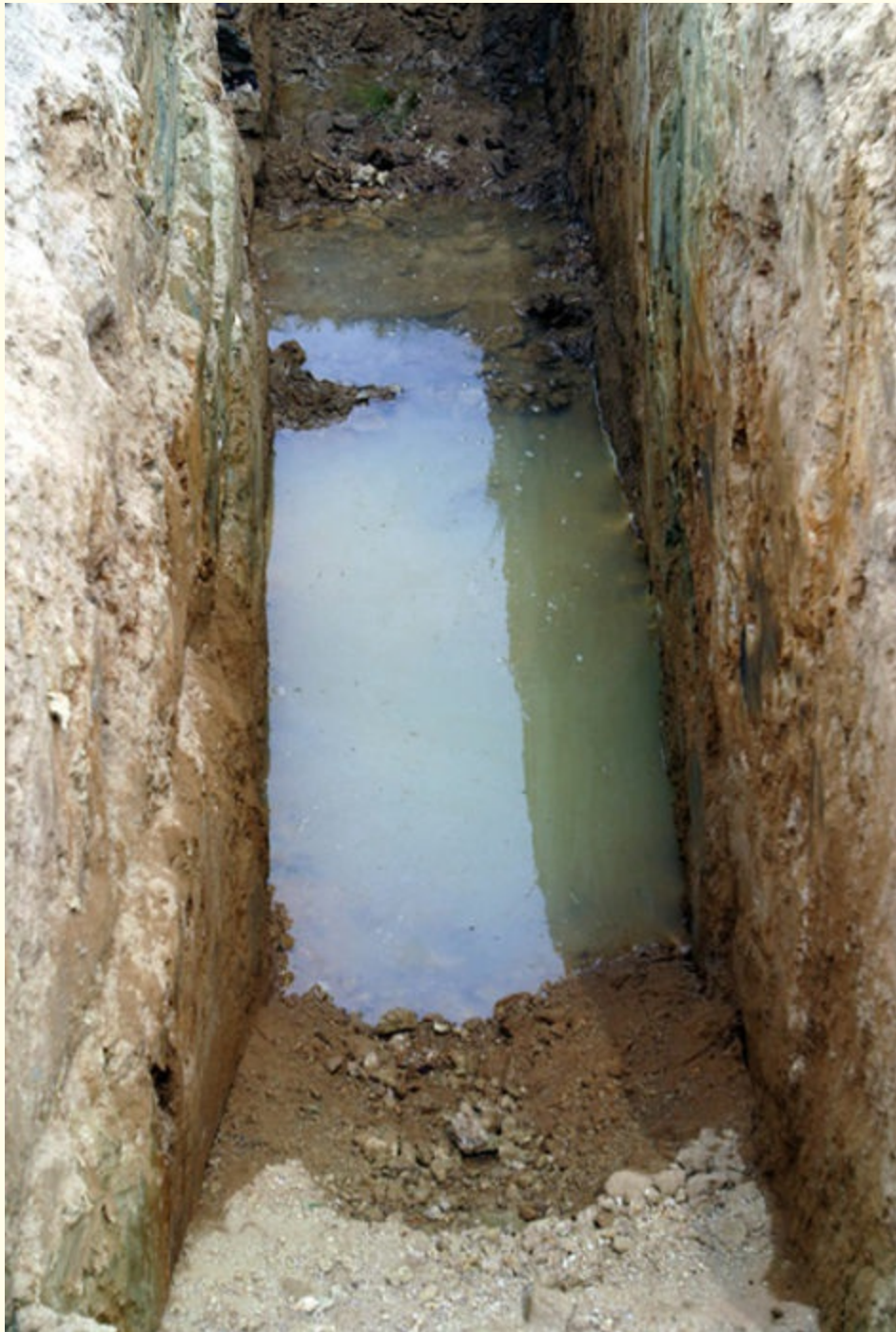
FIGURE 8-7 Water creates extreme forces on trenches that can compromise already poor conditions. Courtesy of Cecil V. "Buddy" Martinette, Jr.
