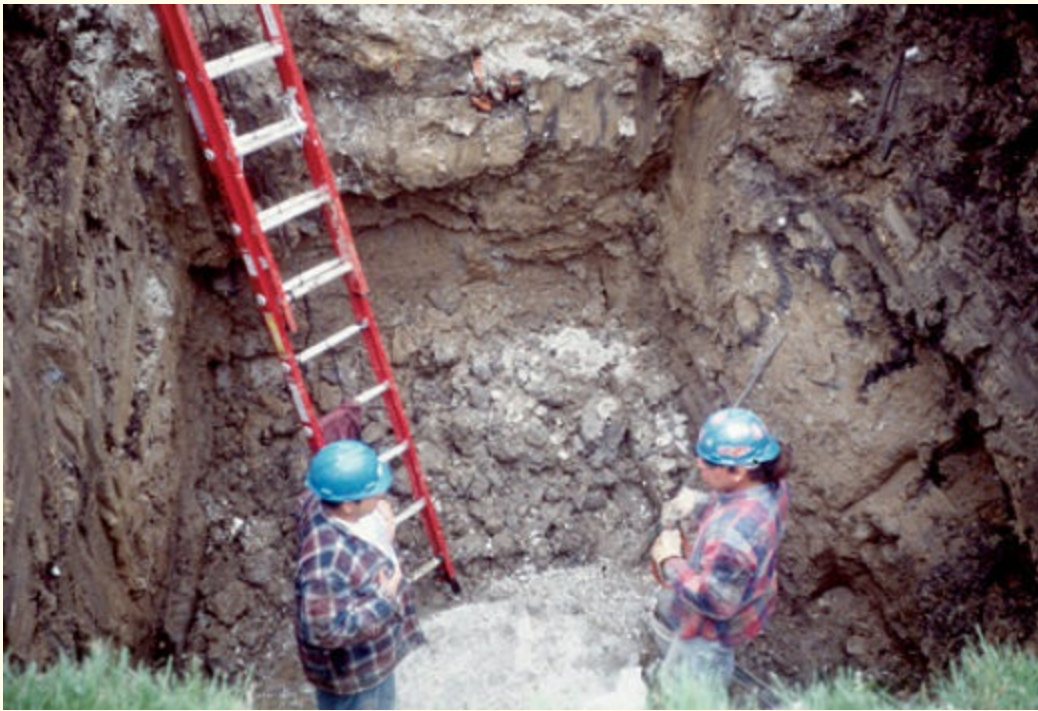
FIGURE 1-4 There will always be workers who do not appreciate the hazards involved with trench work and are willing to take an ill-advised risk.
