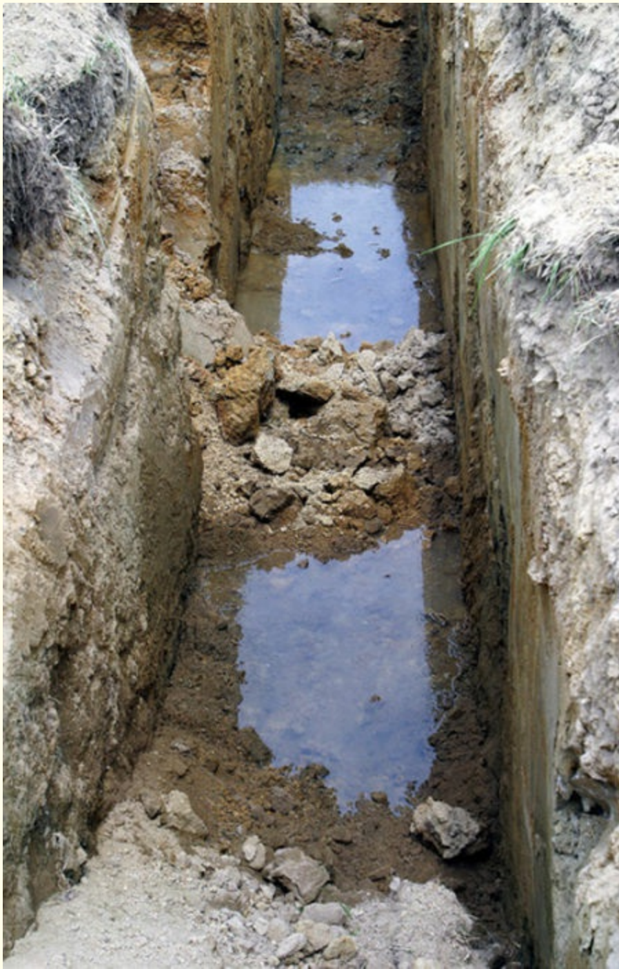
FIGURE 3-10 When running or standing water is present in a trench, the site should always be considered type C soil. Courtesy of Cecil V. "Buddy" Martinette, Jr.
