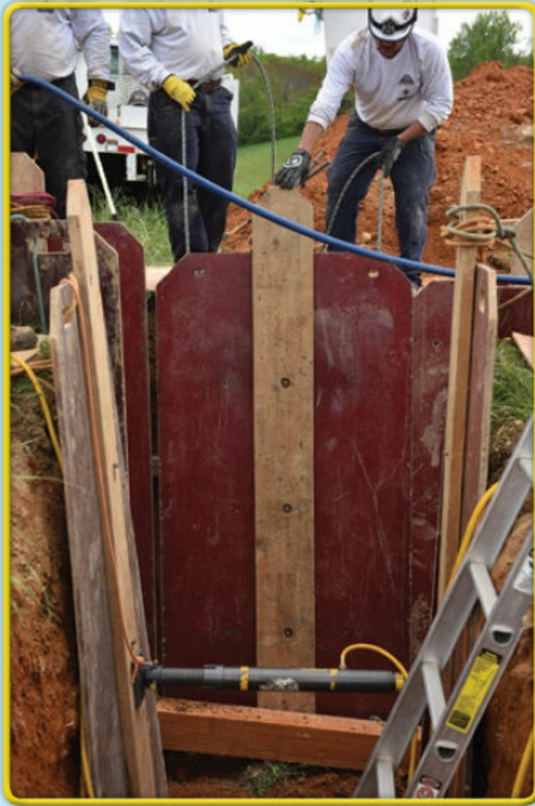
6 Place a panel on the long wall between the two shored panels.
