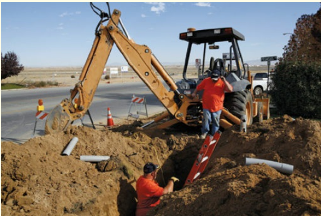
FIGURE 7-4 Most trench work takes place in limited-size openings, and a small area means that you do not have to look long to find the victim.
