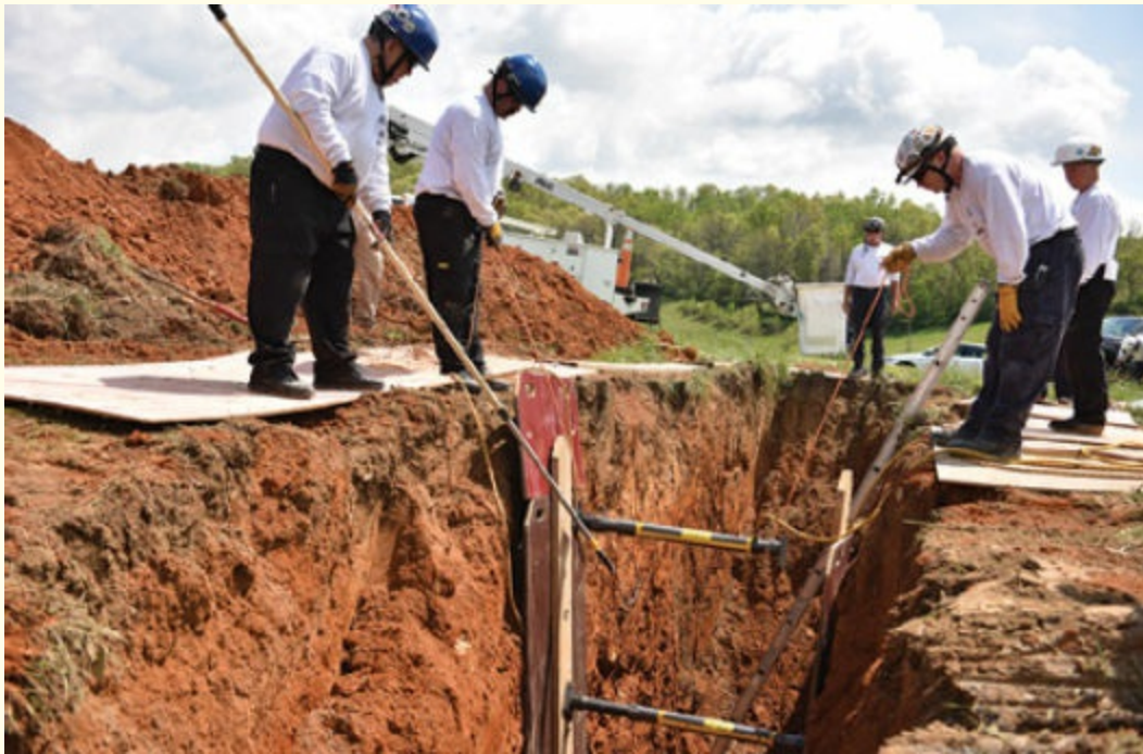
FIGURE 5-5 Make sure that the shoring team members understand the type of protective system desired and are well versed in how to operate your specific type of shores.
