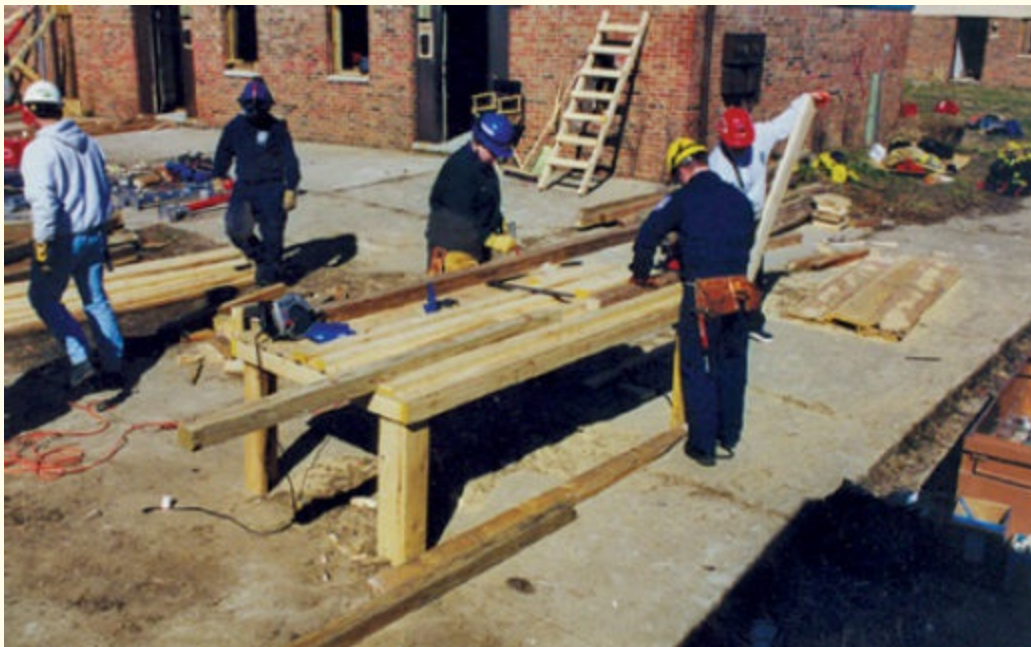
FIGURE 5-3 Building a cutting station on timber trench incidents will save time later in the operation and provide a safer work space for rescue personnel.
