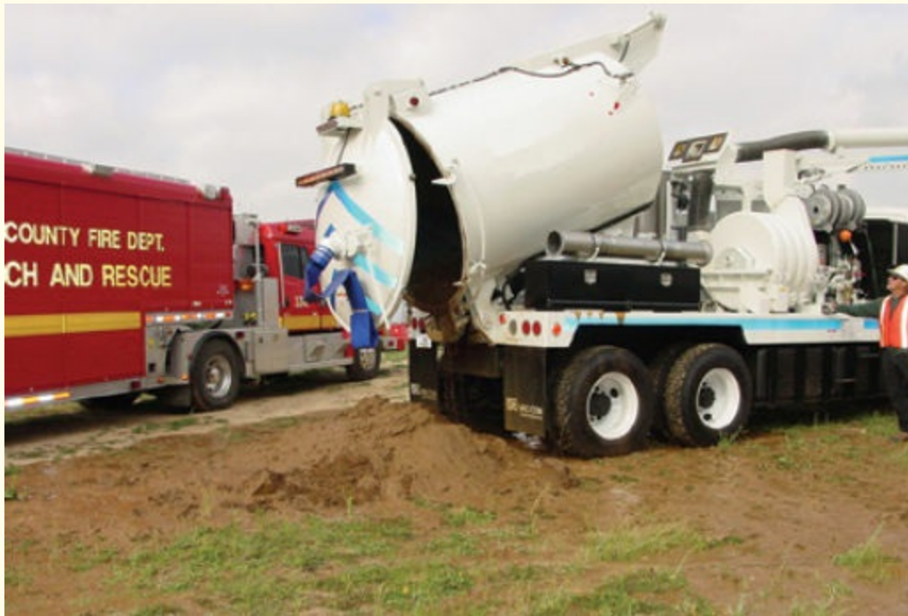
FIGURE 12-8 Municipal vacuum trucks can expedite the removal of soil; however, the soil must be of the proper size and consistency that it can be picked up by the vacuum.
