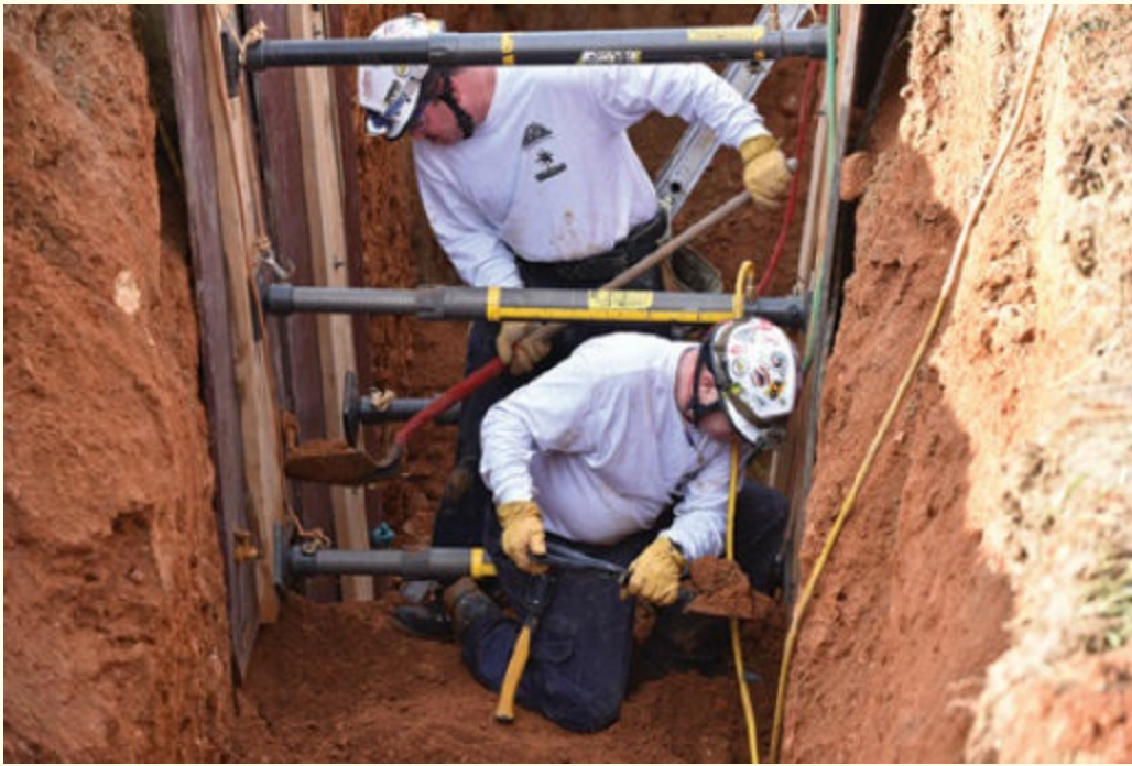
FIGURE 6-19 The entrenching tool is a must for digging in the limited space of a trench.
