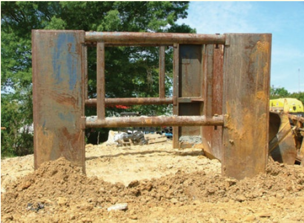
FIGURE 10-18 The trench box is a very stable commercial piece of equipment used to provide worker protection.
