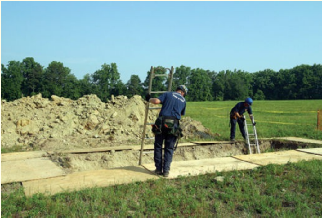
FIGURE 1-8 Always provide rescue personnel with two separate means of egress and ingress to the trench.
