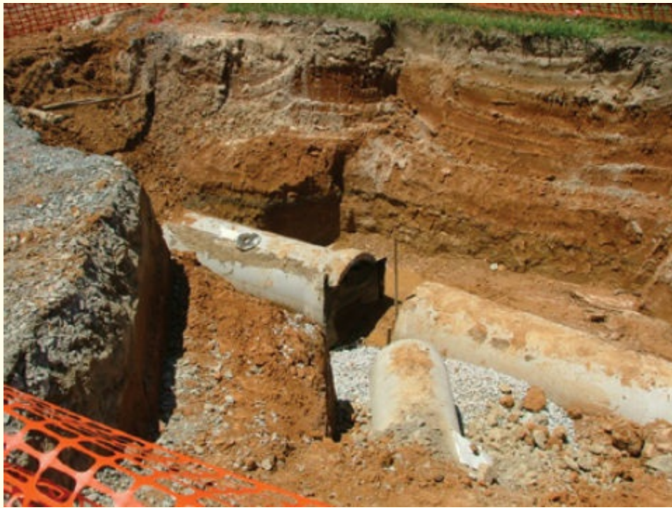
FIGURE 7-1 Large pipes mean deep and wide trenches. Courtesy of Cecil V. "Buddy" Martinette, Jr.
