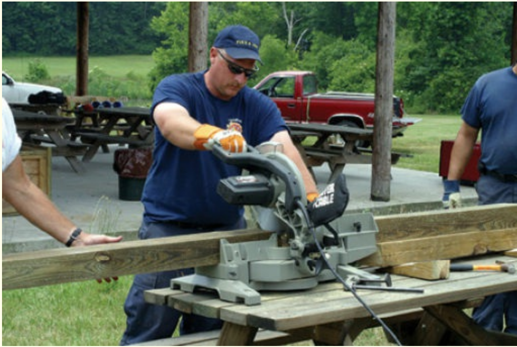
FIGURE 6-13 Wood can be cut to various lengths and used as shores. Wood is also relatively inexpensive and widely available in most communities.
