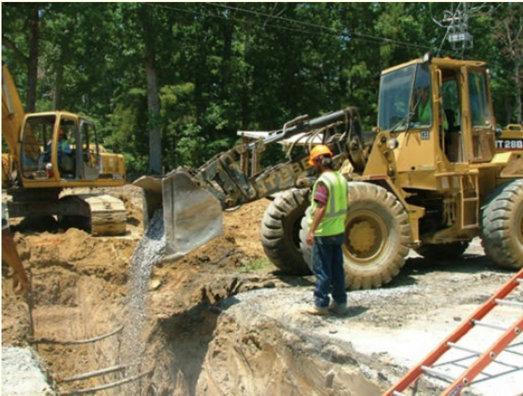
FIGURE 1-5 Heavy equipment operation and final placement can complicate rescue efforts at the scene of a trench collapse.
