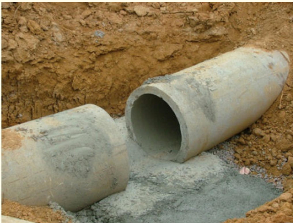
FIGURE 7-5 When conducting size-up, you must consider which type of work was being done at the time of the collapse. Open pipes can provide refuge for victims in a collapse.
