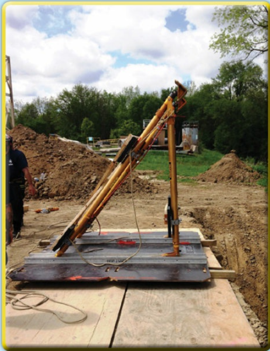
2 Assemble the excavation raker system while working on the lip protection. Courtesy of Ron Zawlocki
