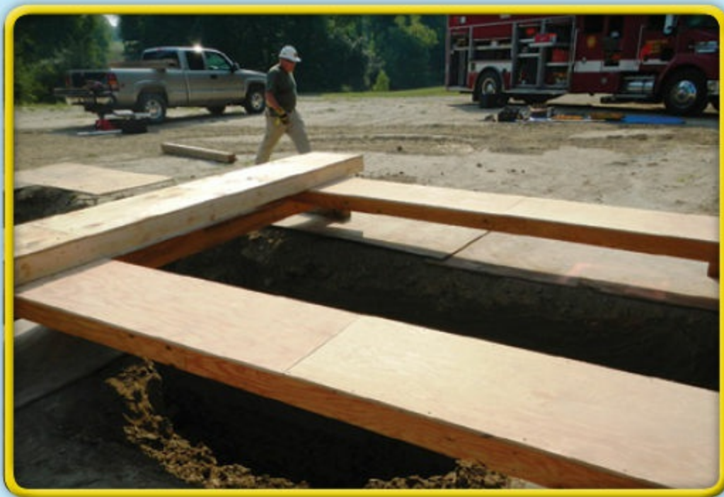
4 Lip bridge over a large wall shear. Courtesy of Ron Zawlocki
