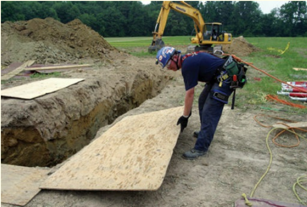
FIGURE 6-6 Ground pads that are 4 × 8 feet in area should be your first choice for trench lip protection.
