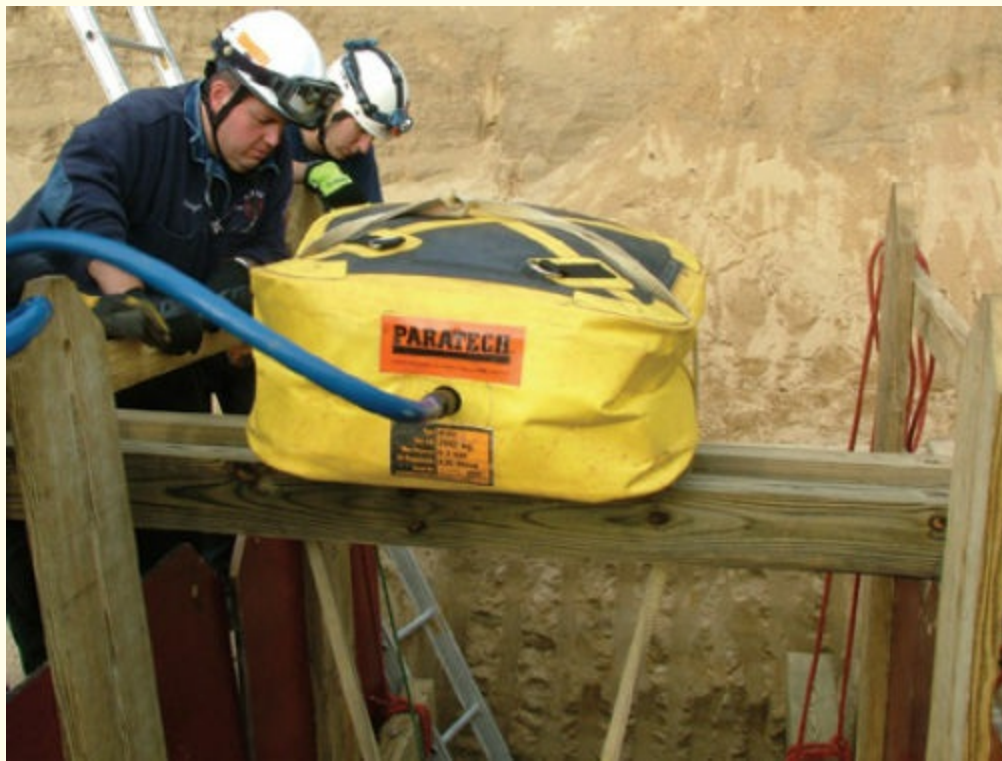
FIGURE 9-18 Low-pressure bag being used to lift an object in the trench. Courtesy of Bob Schilp
