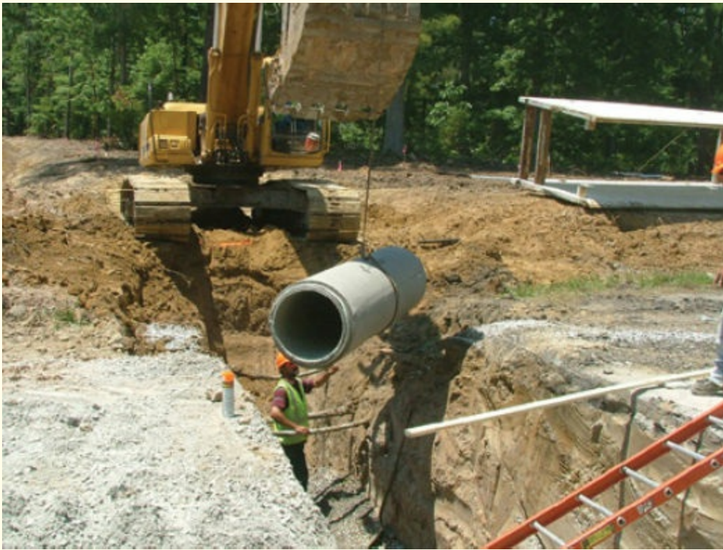
FIGURE 1-6 There are many opportunities for mishaps when using heavy equipment for lifting operations. Courtesy of Cecil V. "Buddy" Martinette, Jr.
