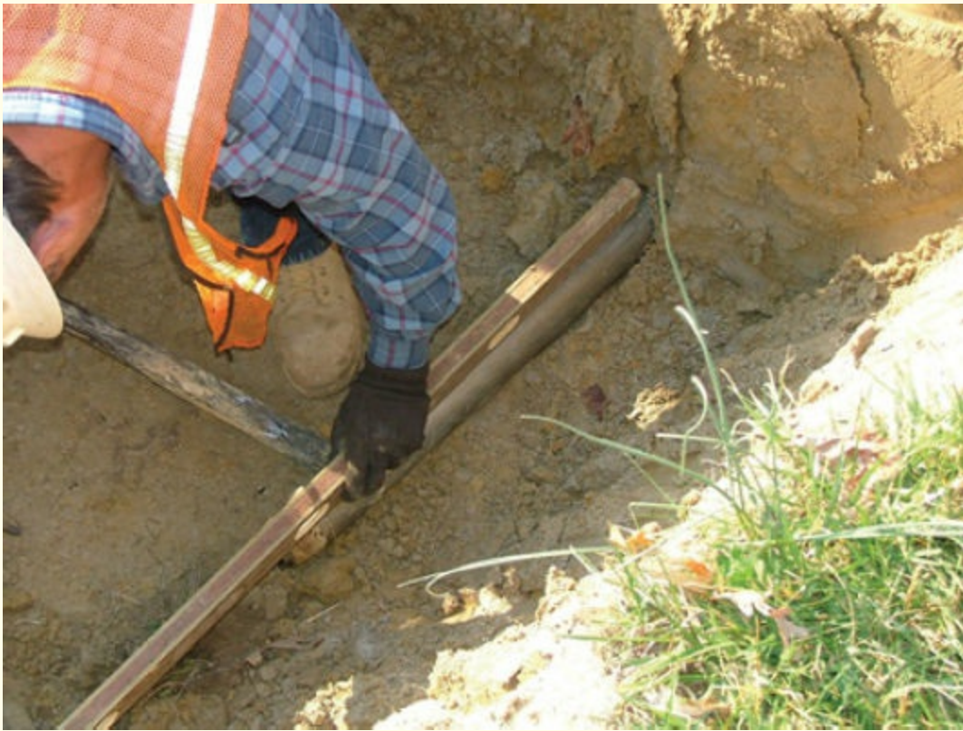
FIGURE 4-10 Piston augers used to get utility lines under roads create vibration, which affects trench and spoil pile stability.
