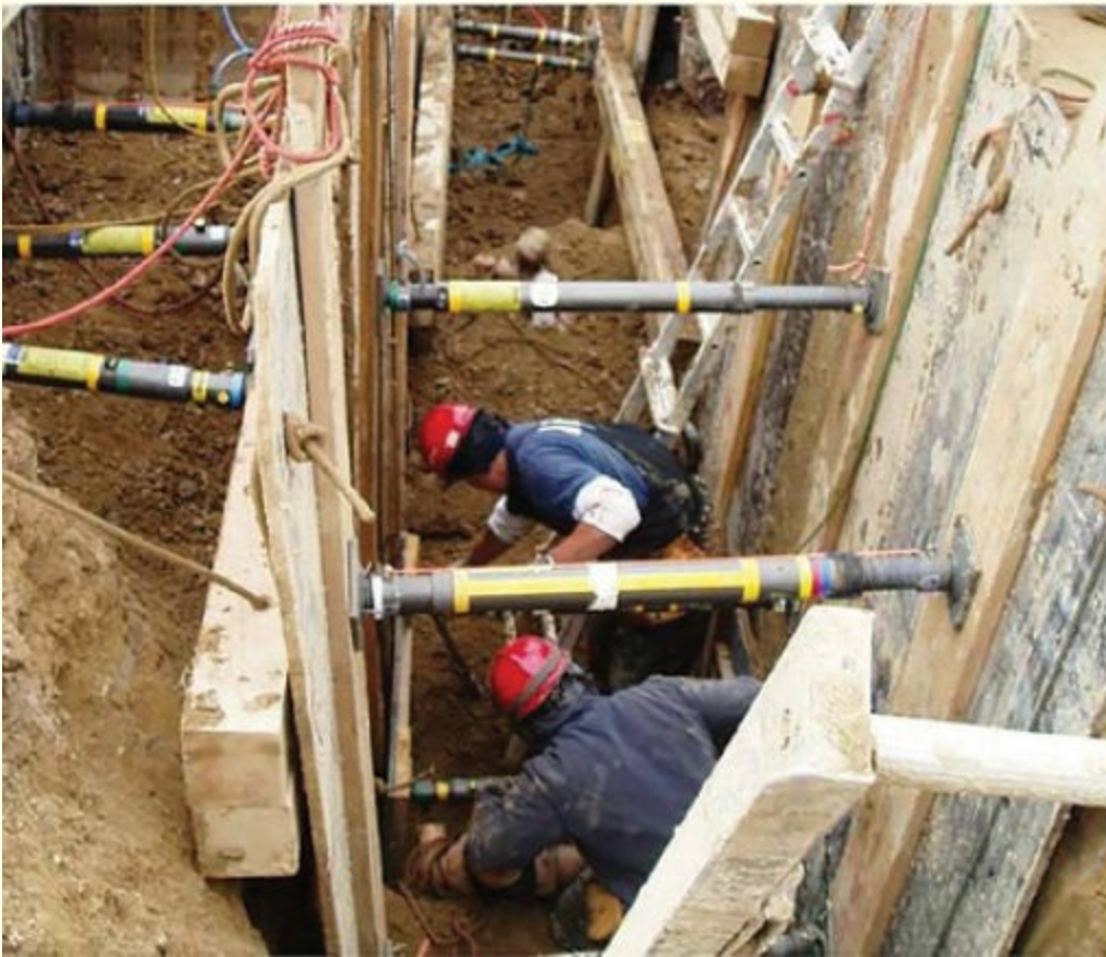
FIGURE 6-18 Advanced shoring techniques include the use of struts to fill in voids.
