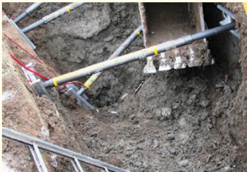
FIGURE 3-6 Rescuers mistakenly considered this active soil to be type A. They used a construction-based shoring technique (spot shores) designed for stable and cohesive soil.
