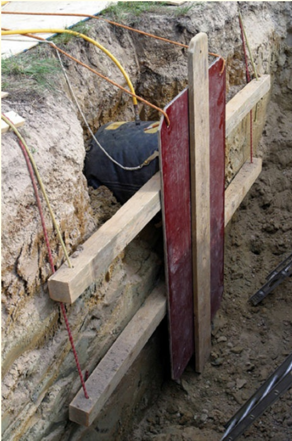
FIGURE 9-14 Air bags have many applications in trench rescue. In this photo, they are used to fill a void in a trench slough.
