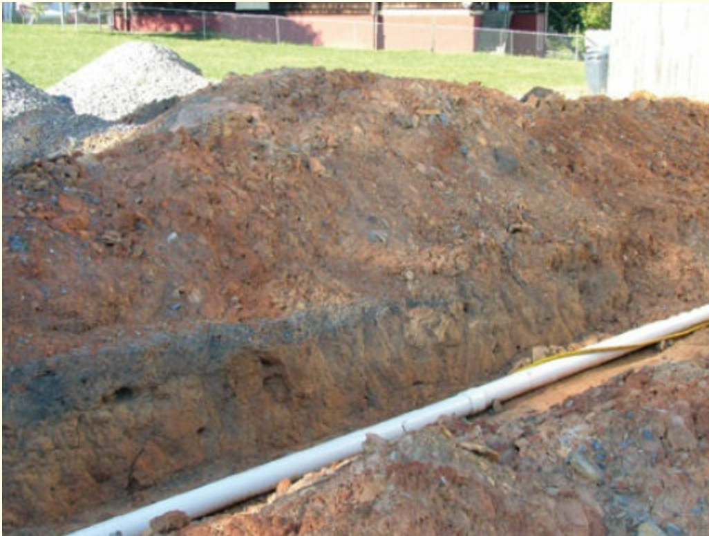
FIGURE 8-4 The spoil pile is frequently placed right next to the trench lip, which creates tremendous forces on the exposed trench walls. Courtesy of Cecil V. "Buddy" Martinette, Jr.
