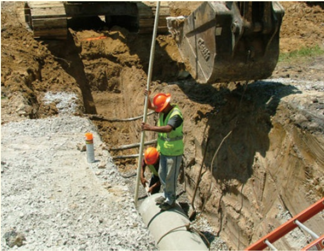
FIGURE 4-3 Workers in unprotected areas of a trench are not an uncommon sight in the construction industry. Courtesy of Cecil V. "Buddy" Martinette, Jr.
