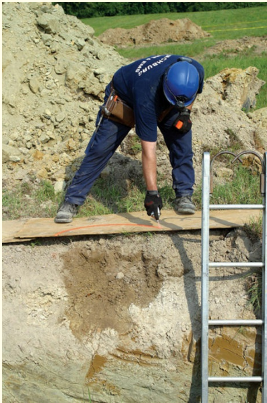
FIGURE 6-7 Marking ground pads communicates to rescue personnel potential cracks or dangerous areas that should be monitored or avoided.
