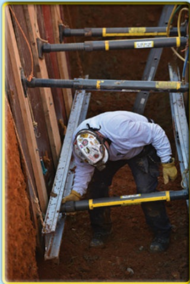
7 Raise the bottom wales and tie them off no more than 2 feet (0.6 m) above the trench floor. Install struts on the wales at
