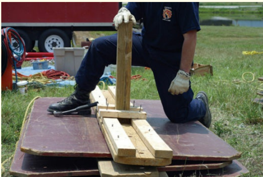
FIGURE 10-11 Railing (stringers) the strongback can make the installation and adjustment of timber shores easier for the shore installer.
