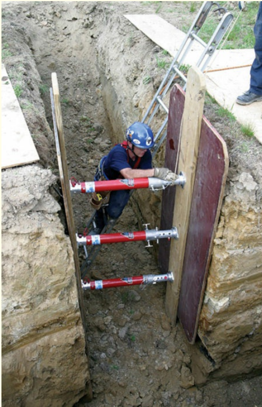
FIGURE 10-8 The top shore completes the installation of the first set of panels.
