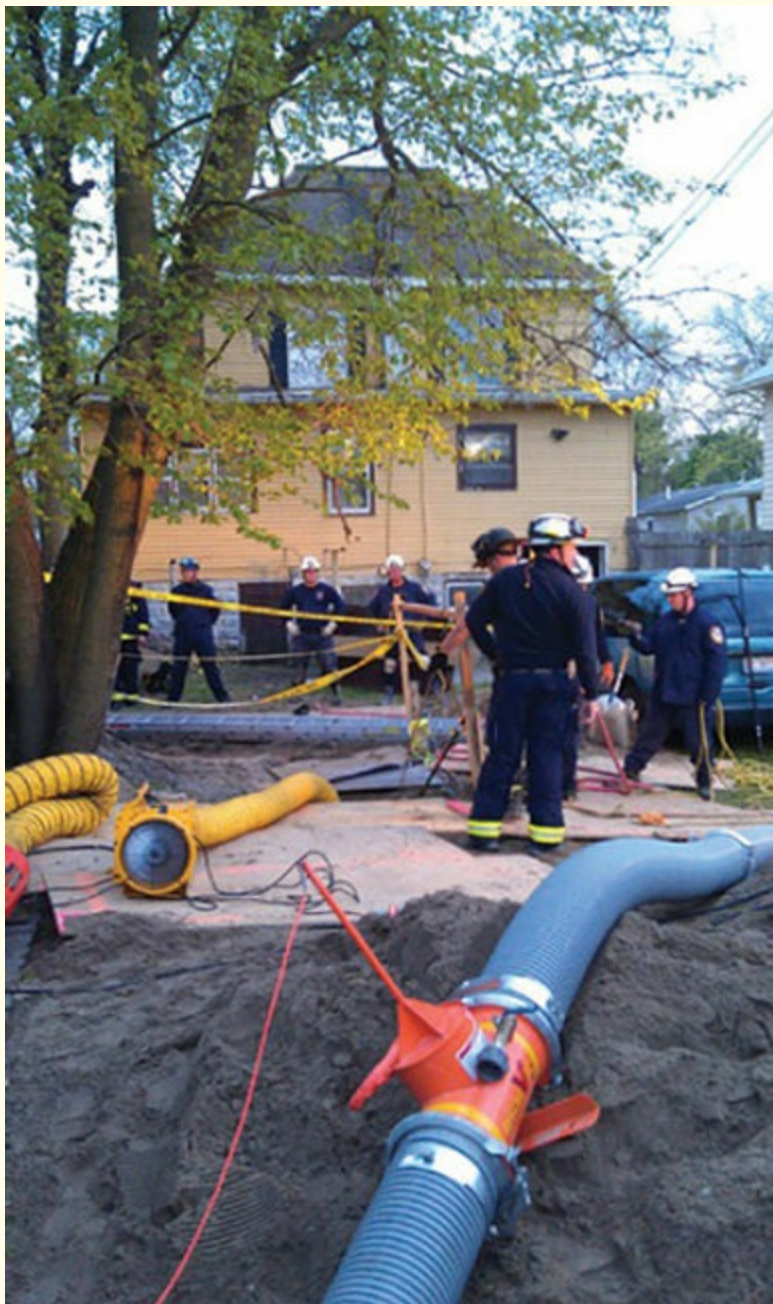
FIGURE 12-11 Technology like the vacuum system combines older municipal vacuum technology with a product specifically designed for rescue personnel and dirt excavation.
