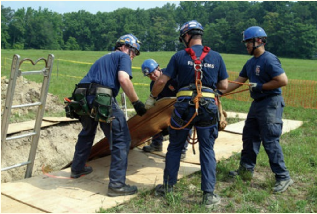
FIGURE 5-4 Panel teams and the techniques they use to set panels are very important to building a functional protective system.
