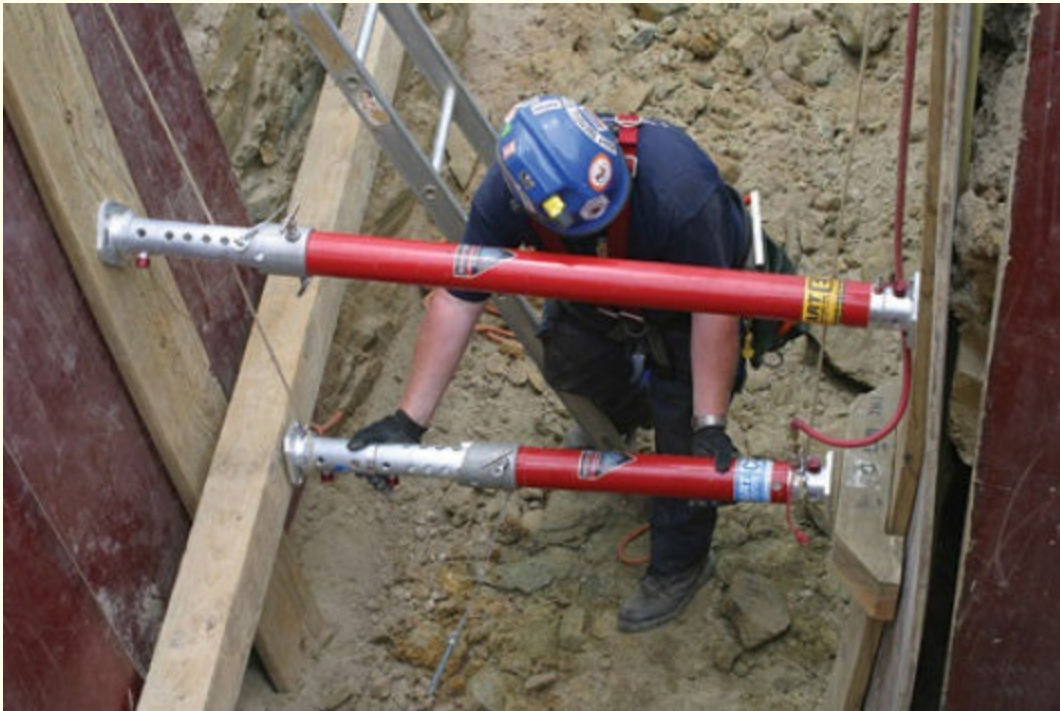
FIGURE 10-10 This style of pneumatic strut has a collar that twists and uses pins to obtain its full strength. Rescuers must minimize their exposure time during installation.
