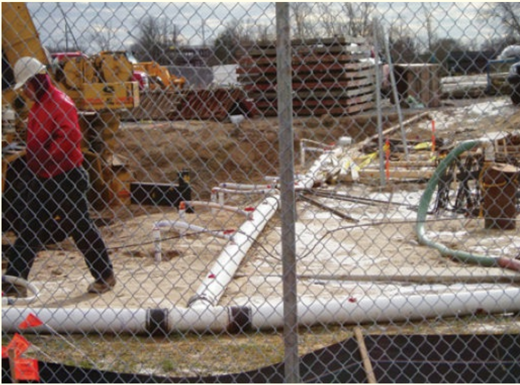
FIGURE 3-11 Look for indications that the area around the excavation has been well pointed. Courtesy of Ron Zawlocki
