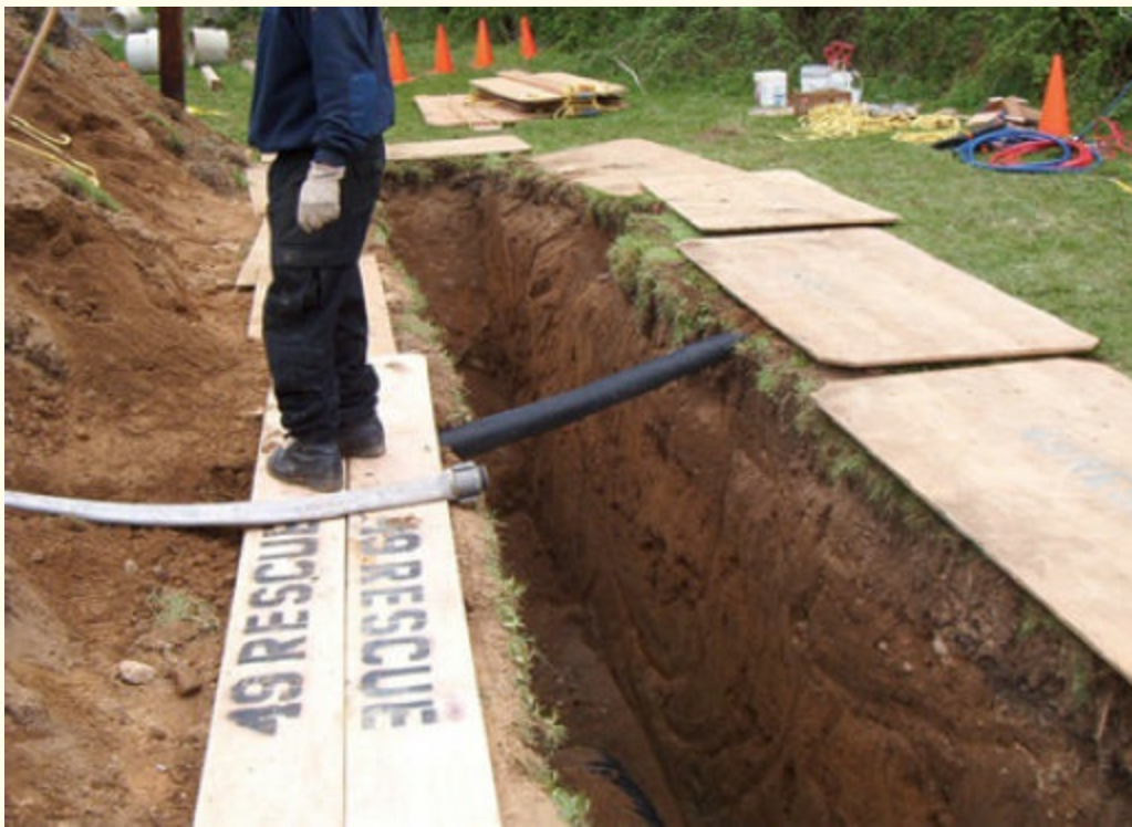
FIGURE 6-8 Used on the spoil side of the trench, the 2 × 12-inch ground pad works well. Courtesy of Cecil V. "Buddy" Martinette, Jr.
