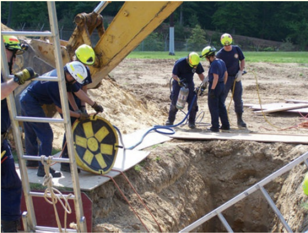
FIGURE 4-9 Rescue personnel need to consider the additional force that heavy equipment adds to the trench protective system requirements.
