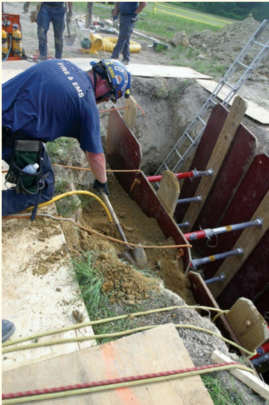
FIGURE 11-4 Voids can be filled with dirt when air bags will not work or are not available. © Jones and Bartlett Publishers. Courtesy of MIEMSS.
