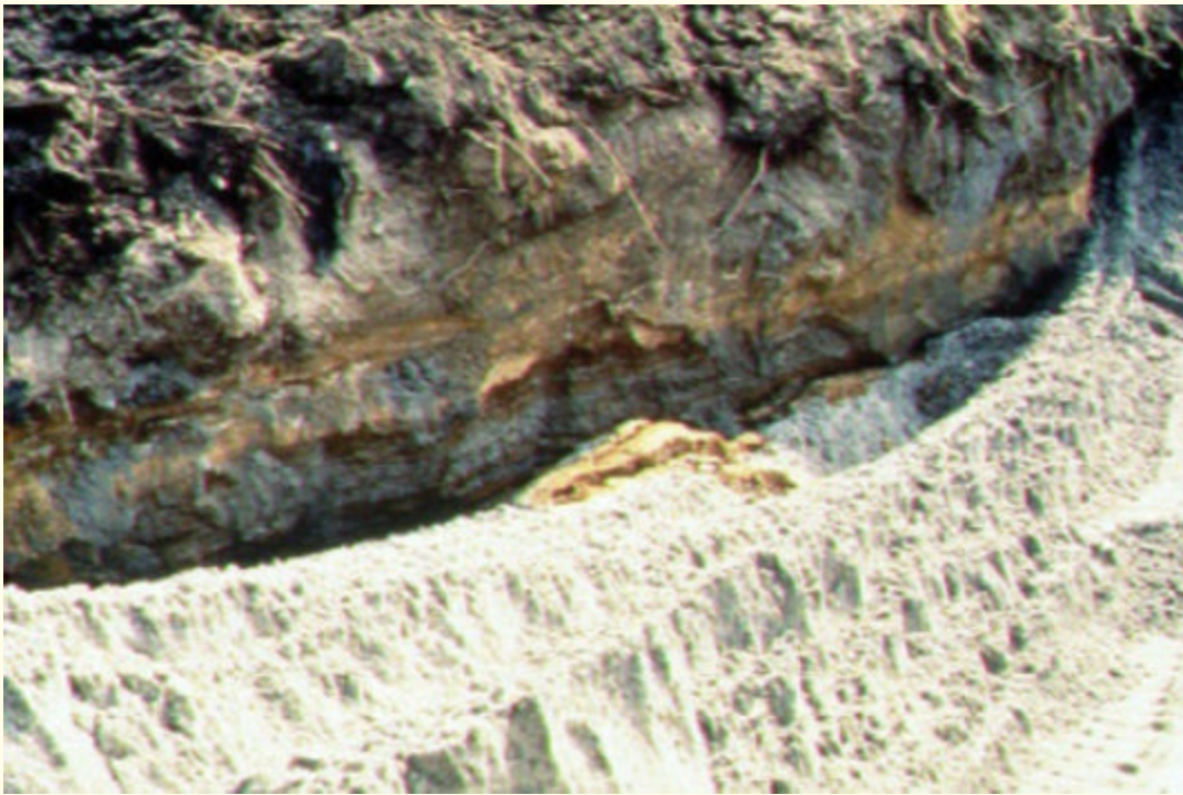
FIGURE 3-8 Be very cautious of layered soils in an open trench. Courtesy of Cecil V. "Buddy" Martinette, Jr.
