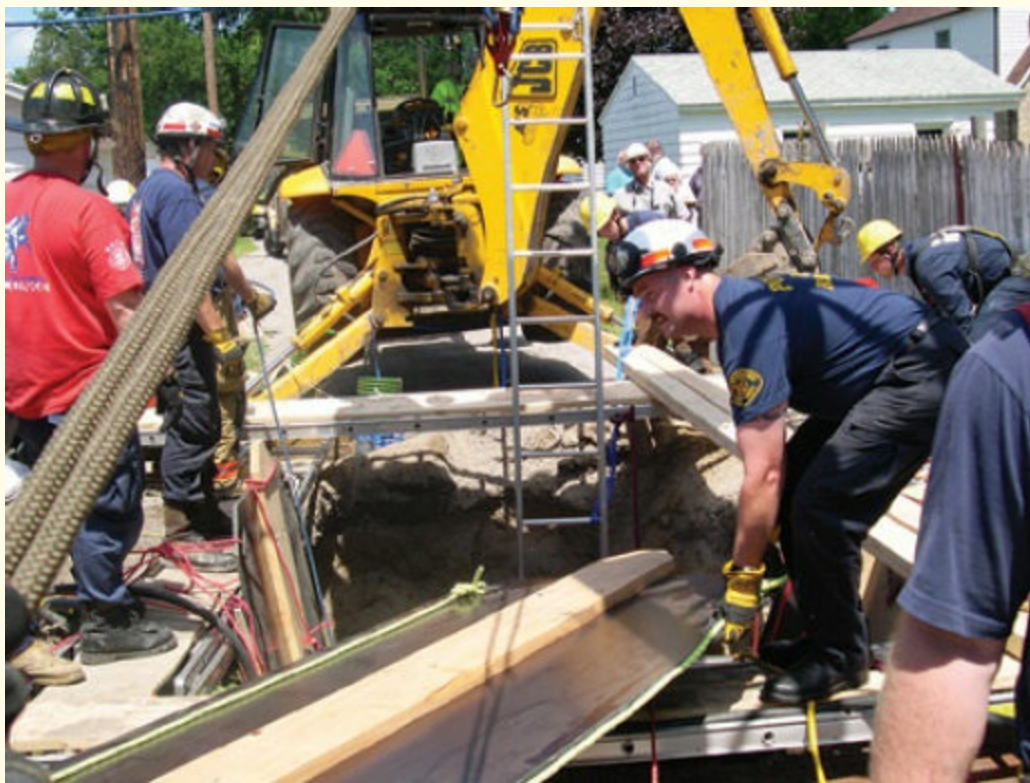
FIGURE 10-1 This four-sided lip bridge was needed to install shoring over a repair hole where three walls collapsed on a city worker.
