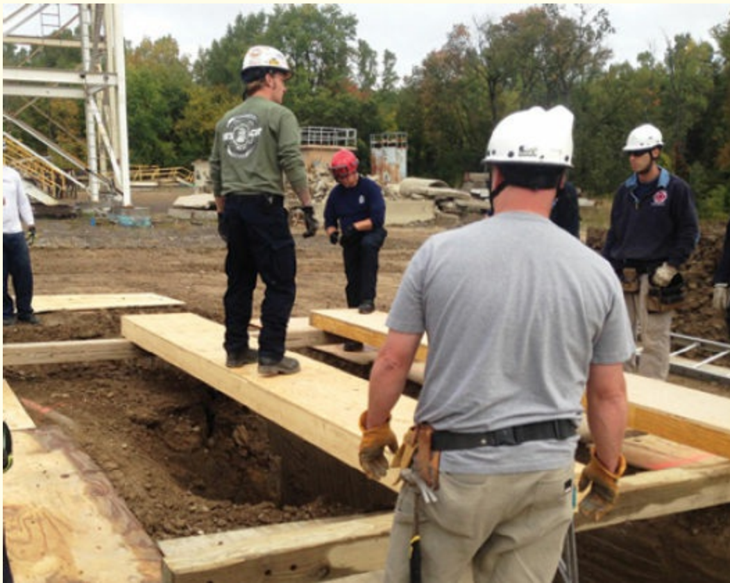
FIGURE 6-9 This lip bridge is used to work directly over a large lip shear collapse. It keeps the rescuer's weight off the missing or damaged wall.
