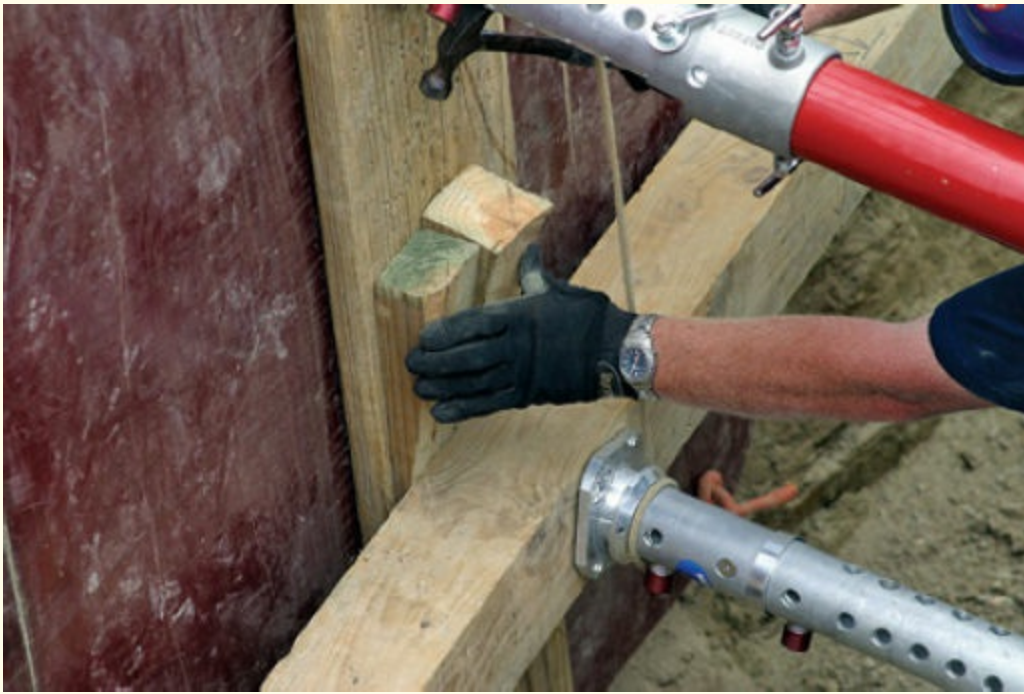
FIGURE 9-23 Wedges being used to fill a void between the wale and the strongback.
