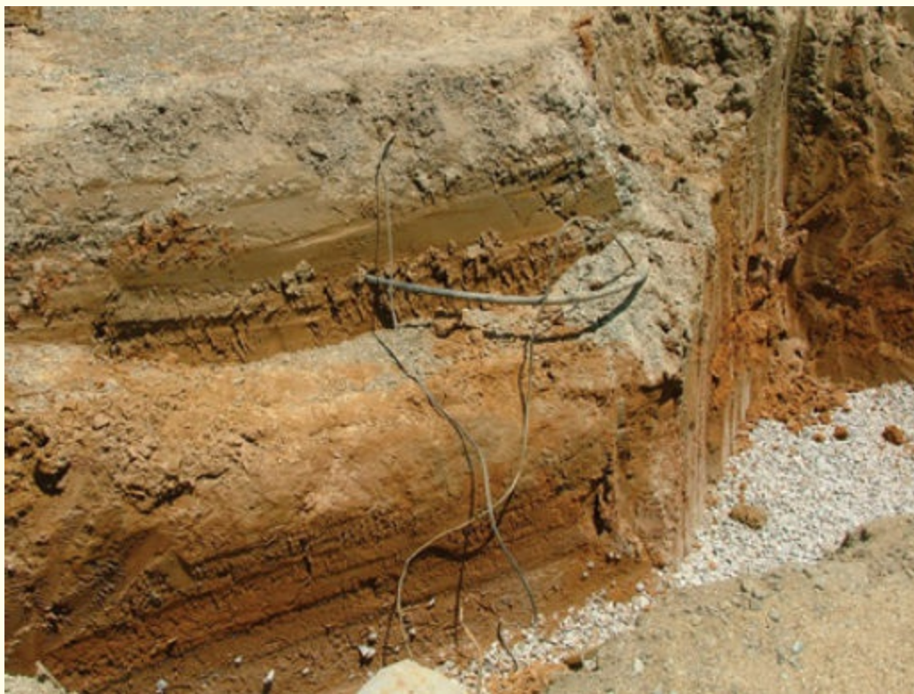
FIGURE 8-5 Electrical hazards should be secured in both the general area and the rescue area. Courtesy of Cecil V. “Buddy” Martinette, Jr.
