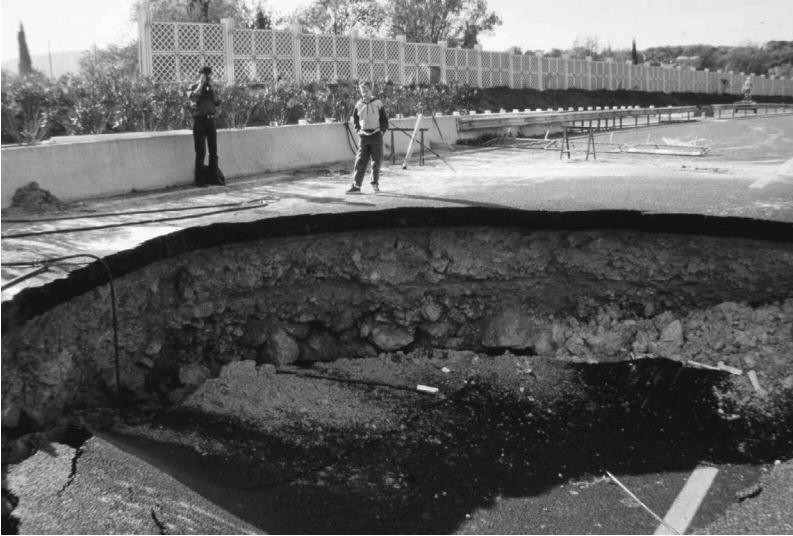
Figure 122. Cannes-Grasse highway collapse (Alpes Maritimes, France) in 1998. The damage was a result of gypsum in the underlying rock being rapidly dissolved due to groundwater pumping to irrigate a golf course.
