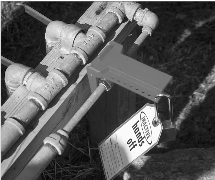
The common process of locking out and tagging a simple in-line valve could save someone's life.
