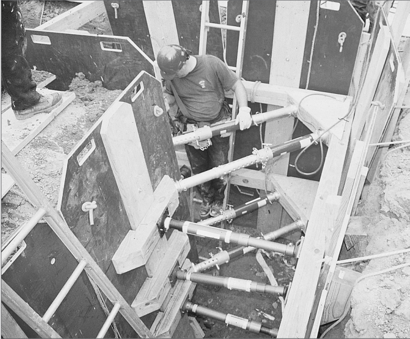
Trench operations are closely linked to engulfment scenarios. Here, during a training exercise, shoring jacks and boards are being used to hold back the earth.
