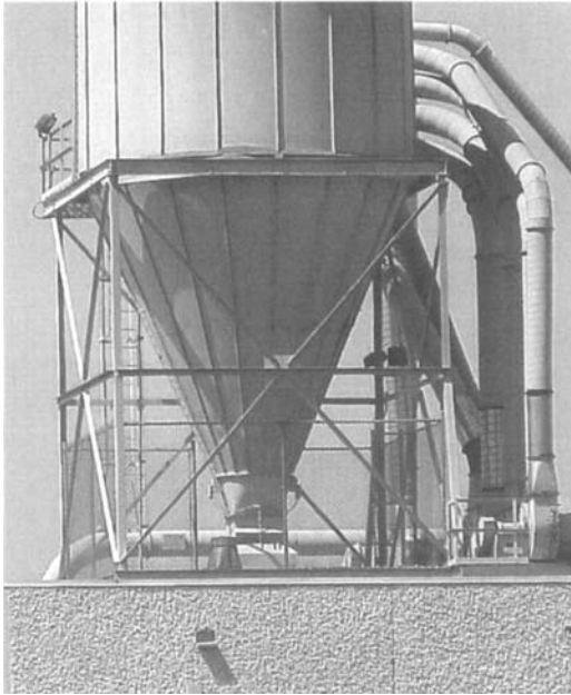
Figure 1.12 Confined spaces having configurations that could trap or asphyxiate an entrant are considered permit-required.
