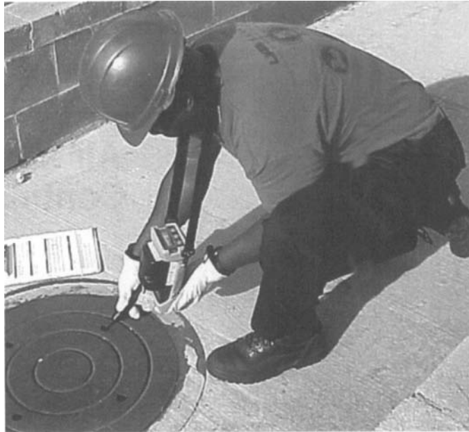
Figure 4.1 The atmosphere of a confined space must be assessed from outside before entry is made.
