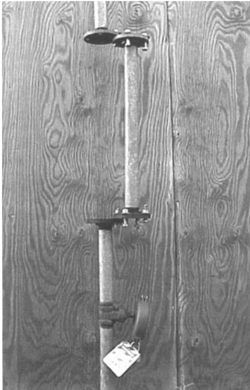
Figure 6.23 Line breaking can be used to isolate a space from contents of pipes, tubes, or ducts.
