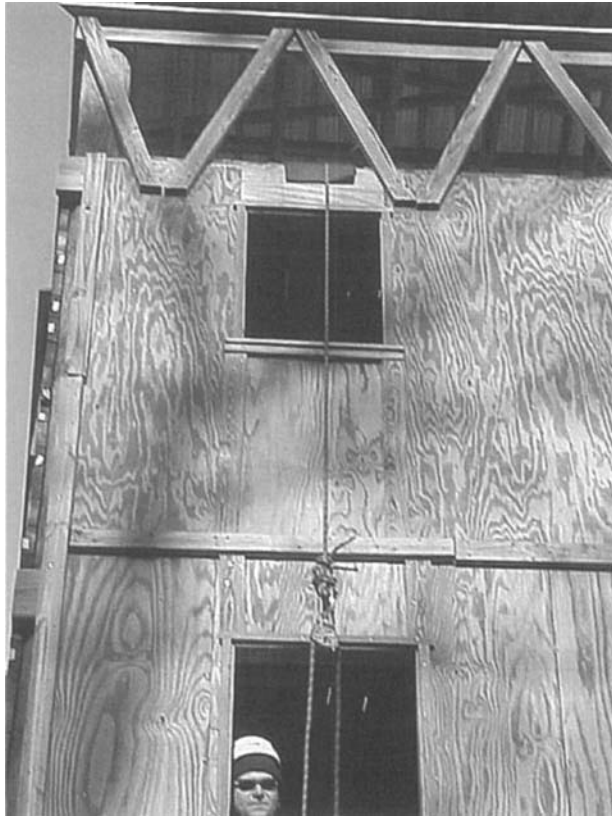
Figure 13.34 Anchor points can be extended to locations where points of attachment are needed but no suitable anchor points exists.
