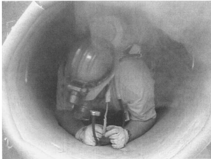
Figure 14.14 Claustrophobia is one hazard of confined space entry.
